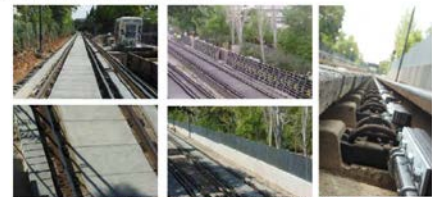
Figure 3 - Mitigation measures (all solutions) at the Athens Metro Line 1 test site: left, horizontal panels; "sound barrier" panels; middle, noise barrier with vertical absorbing panels; right, rail dampers installed
